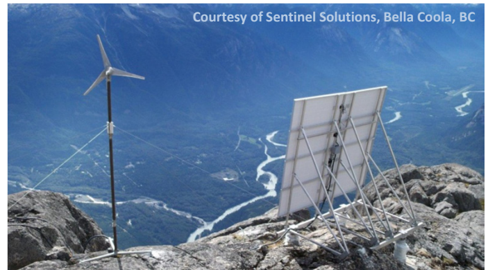
Solar Power and Wind Turbine Deployment British Columbia, Canada
