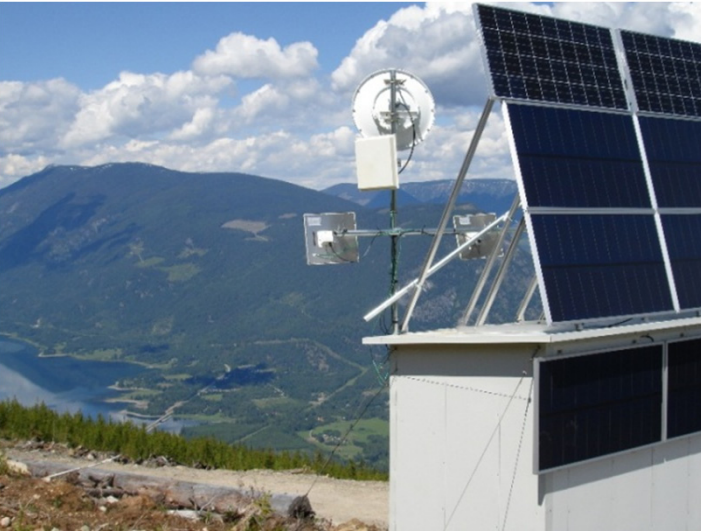
Solar Powered Remote Communication Tower British Columbia, Canada
